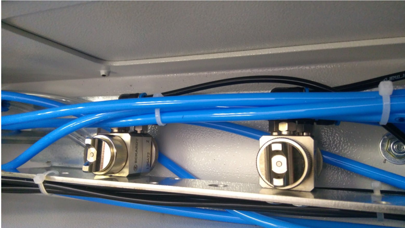
Spray nozzles with feed lines
