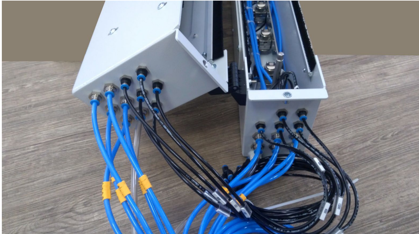
Spray lubricator opened
